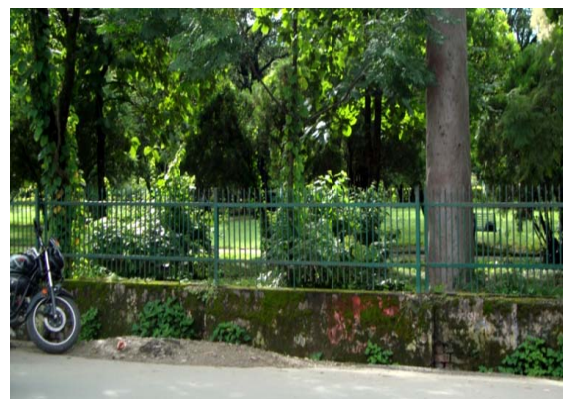
Fig. 10: Poorly maintained boundary wall of park, Dehradun
